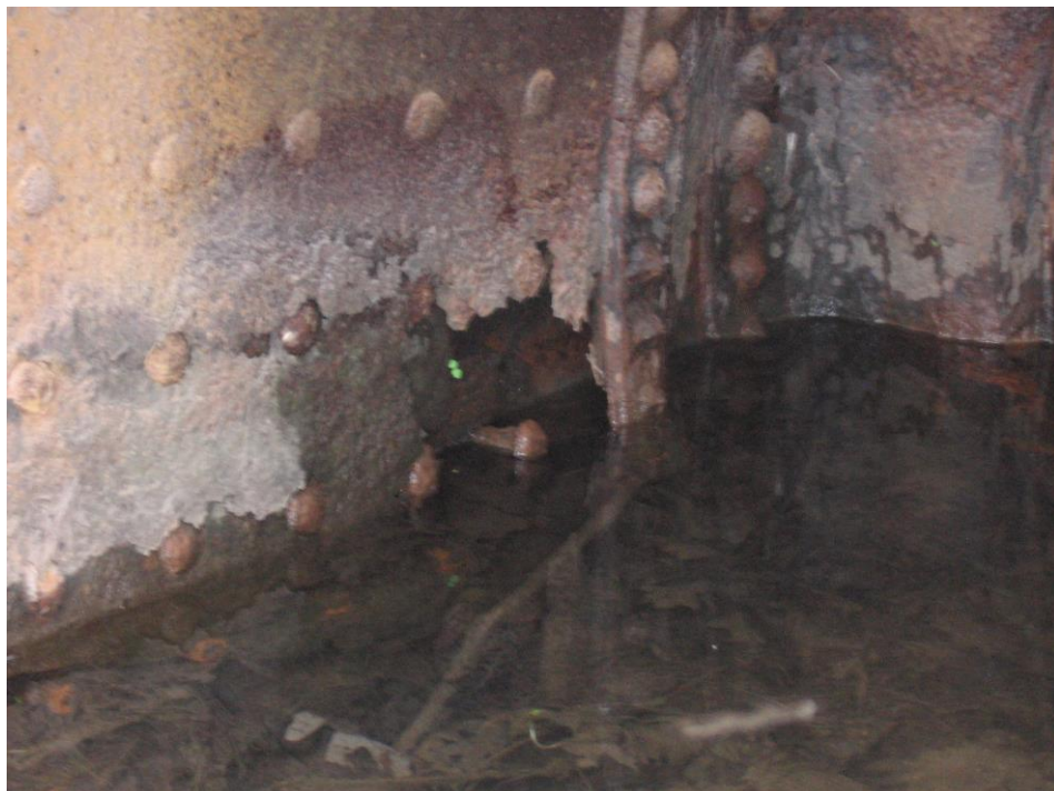
Deterioration of Bottom of Existing culvert
