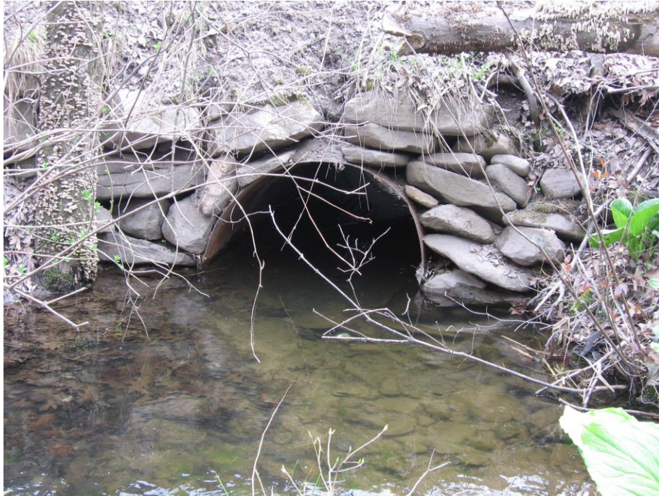
Upstream end of existing Culvert (note deformed pipe opening)
